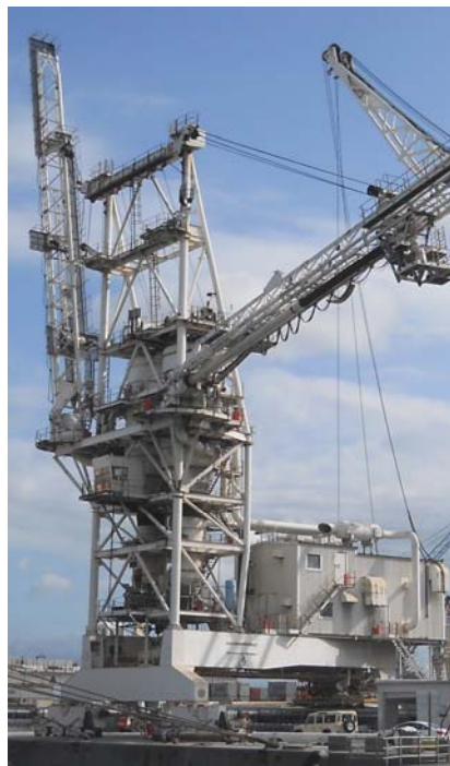
The condemned crane - in danger of collapsing
