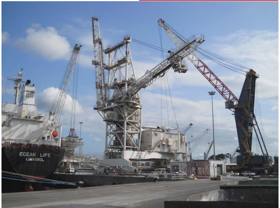
The condemned 460 ton Hitachi crane (centre) that Lovemore Bros had to remove before the burnt out crane could be replaced. Note the two booms (one extended and one upright) weighing 40 tons each that had to be cut off
