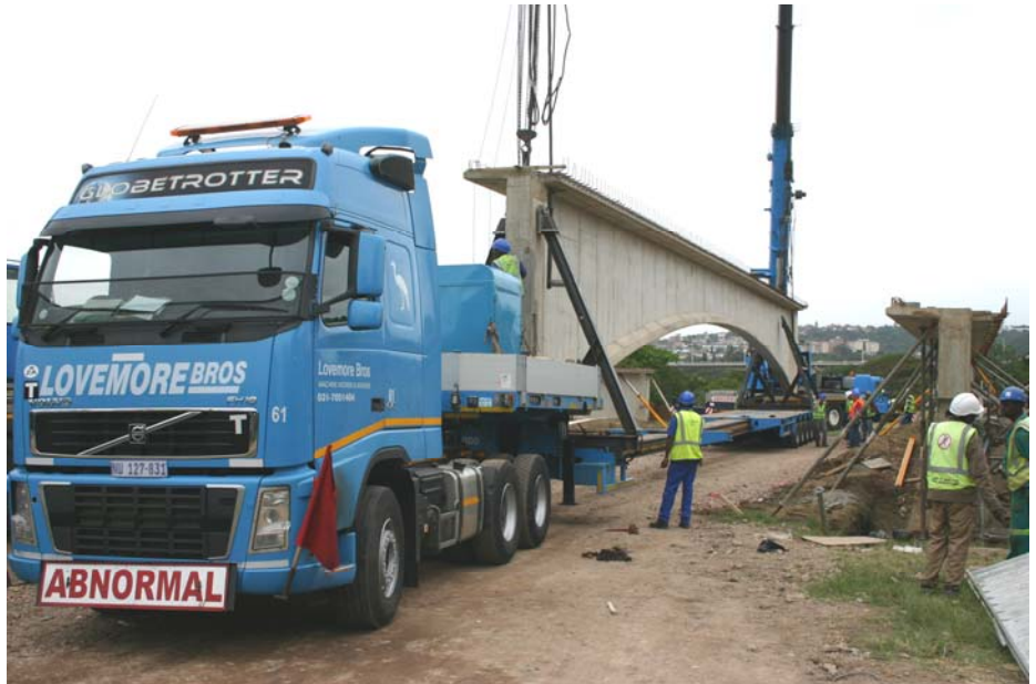
The first of the 15 concrete spans – each about 31 meters long and weighing about 55 tons - fabricated on this vacant land at the end of Riverside road, sets off on the short but hectic journey to the Ellis Brown Viaduct
