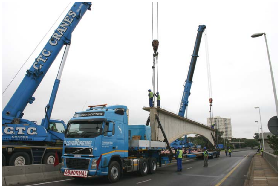
Having arrived safely on the Ellis Brown Viaduct, Lovemore Bros riggers prepare to hoist the span off the trailer and lower it onto the piers
