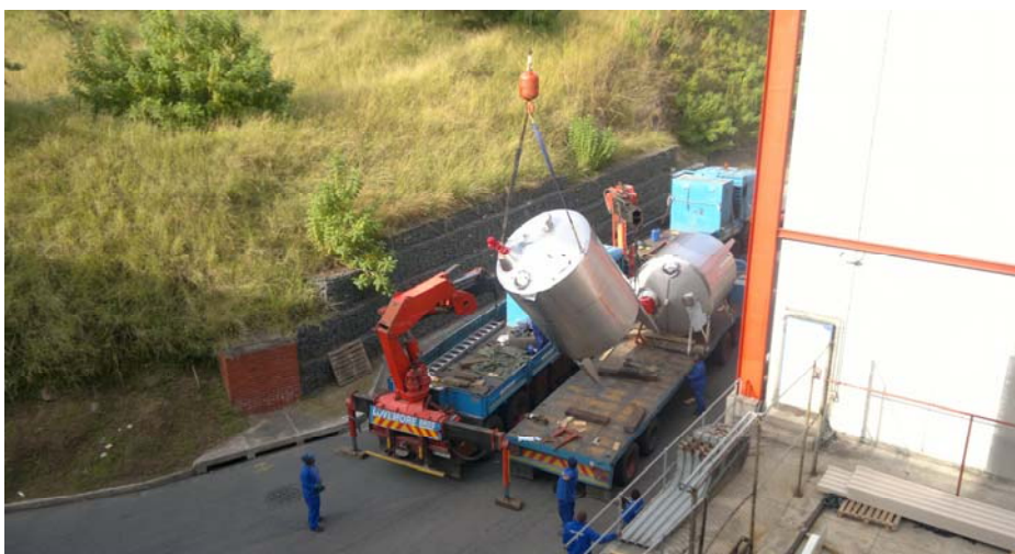
Riggers and crane operators start the tricky maneuvering required to install the new stainless steel tanks at the Ola Ice Cream factory in Queensburgh, Durban
