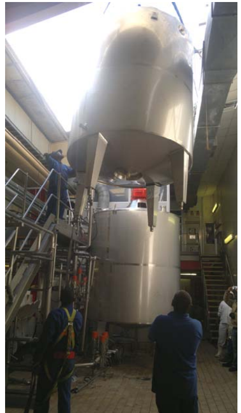
Tight squeeze. Note the narrow gap between the roof girders at right and the catwalk on the left
