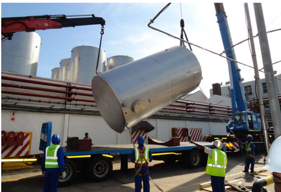
Using the "top & tail" method, riggers guide the two crane operators who gently raise one of the tanks off the flatbed trailer for positioning in the tank farm
