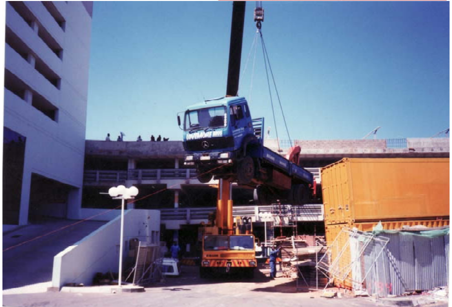
A crane hoists a Lovemore Bros truck to the rooftop of Musgrave Shopping Centre where it was deployed to position the dome
