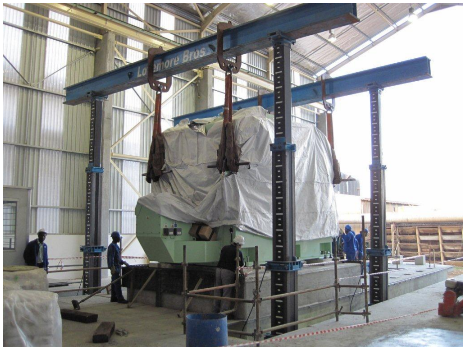
Suspended from the gantry, the generator is gently lowered onto the concrete slab
