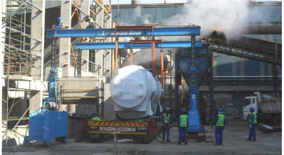
Phase 1 of the project was to rig the 43 ton condenser into position on plinths 3,5 metres above ground level using a 200 ton LPG powered mobile gantry. This was achieved using a cross travel purpose built system to traverse the condenser load
