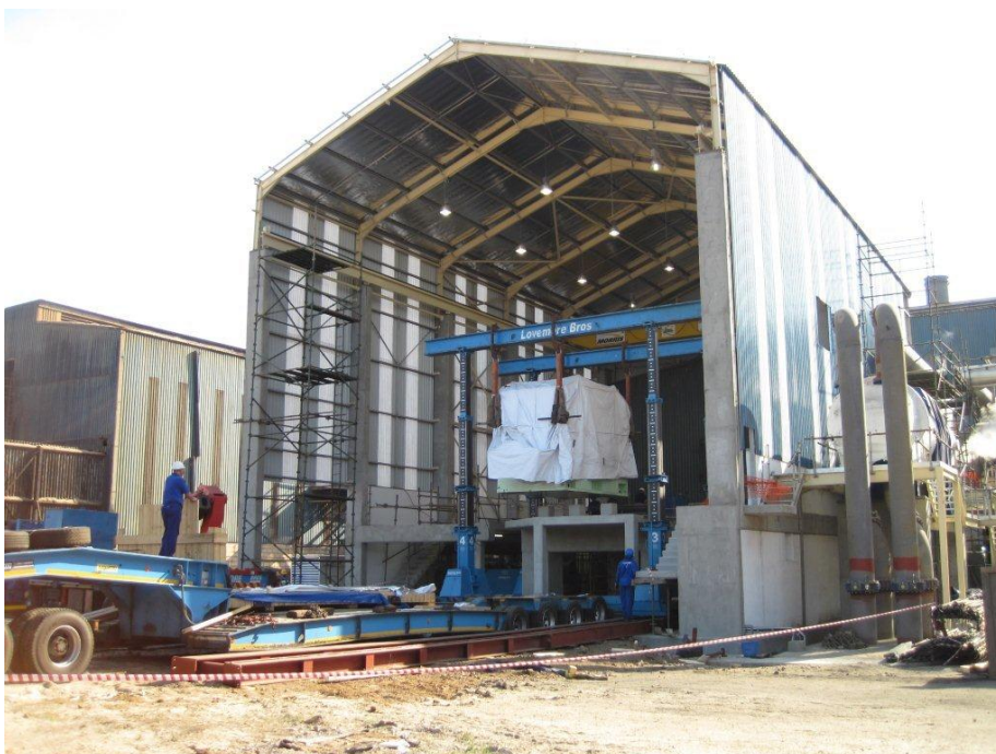
Phase 2 was to place the generator, turbine and gearbox onto a concrete slab 3,5 meters above ground level
